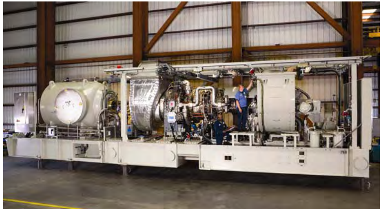
Figure 3. Titan 250 Compressor Set Package
