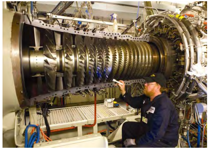
Figure 11. Split Compressor Casing
