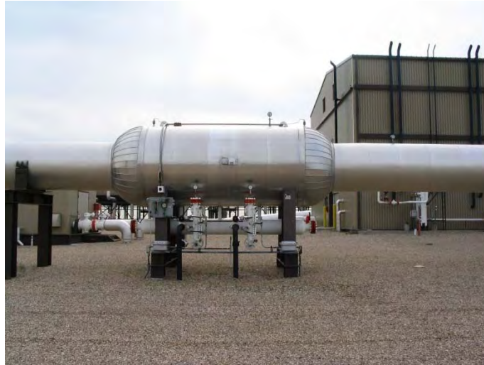
Figure 11: Scrubber at Station #1.
