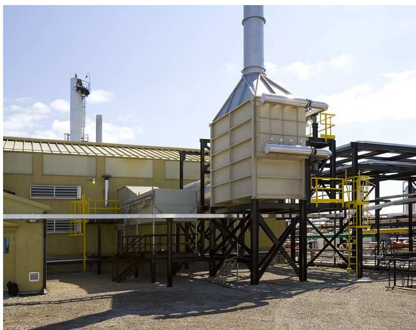
Figure 2 Waste Heat Exchanger
