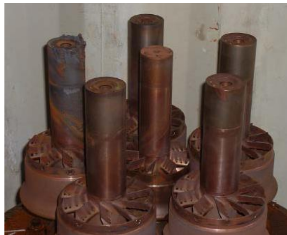
Figure 5: Fuel nozzle damage due to flashback [2]
