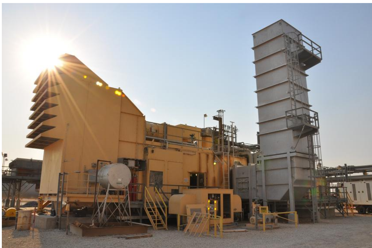
Figure 2: Turbine 'A' package at DCP Goldsmith plant
