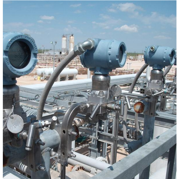
New field transmitters for the driven compressors
