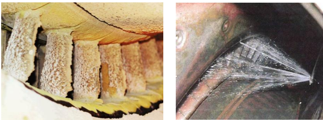
Figure 11: Ash Deposits caused by Crude Oil contamination
